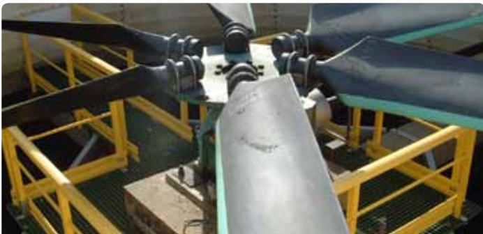
Entrance platforms Cooling tower
