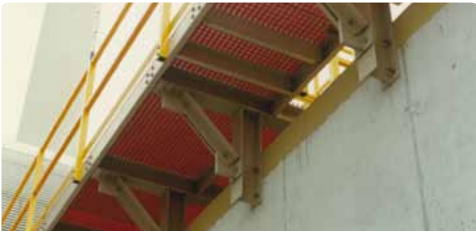
Platform Power plant
