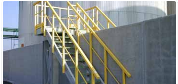
Step over platform Chemical tank storage
